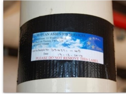
Asbestos marked pipe, Source: UEFG
