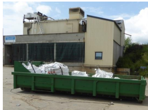
Container with asbestos waste, Source: A2Conseils sprl
