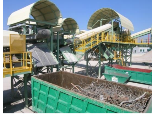
C&D waste recycling plant, Source: ANPAR
